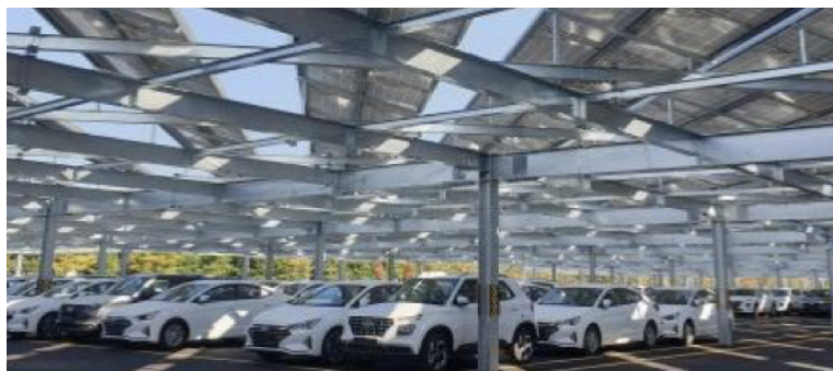
(From the top) Photovoltaic power generation in Hyundai's plant in India 2MWh ESS at Ulsan plant A solar energy facility in the Ulsan factory parking lot
