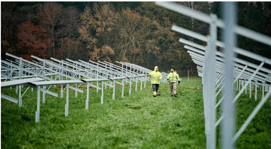
Start of construction for the 6.5 megawatt solar park in Dallgow-Döberitz: A total portfolio of 1.1 GWp will be built by 2026 (symbol photo). (Photo: Christian Horn for SUNOTEC)
